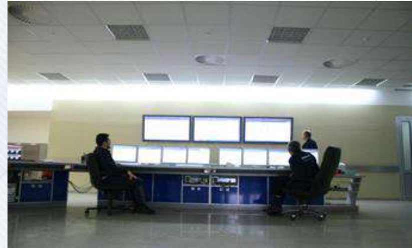
Thermal Power Plant – DCS Control Center
